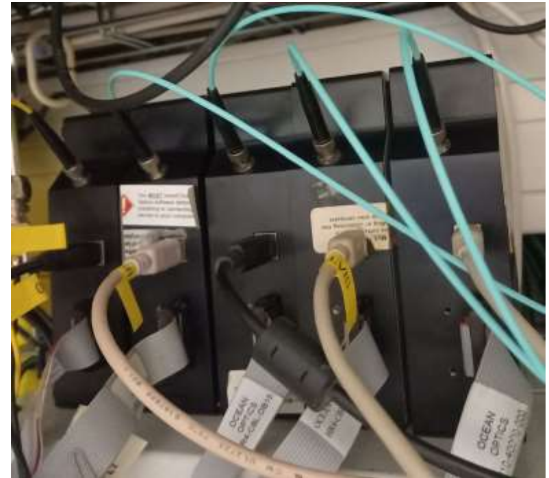
Spectrometers at GOLEM connected with the tokamak via optical fibers
