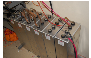
13500 fd, 1300 Volt, 11500 Joule Oil-Filled Energy Storage Capacitor
