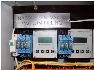
TMP I & TMP II control system
